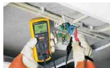
Wiring test in a small distribution box – all in one spot
